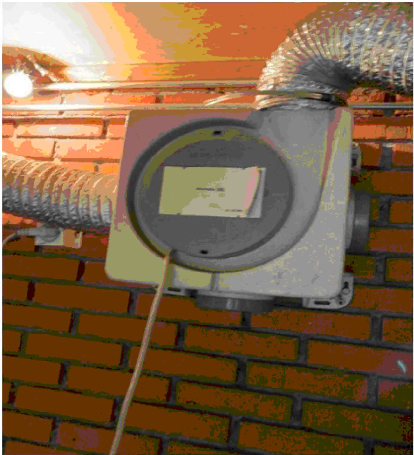
Ventilator TR achter
